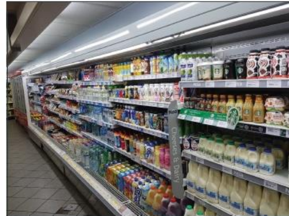
2x large open chillers
